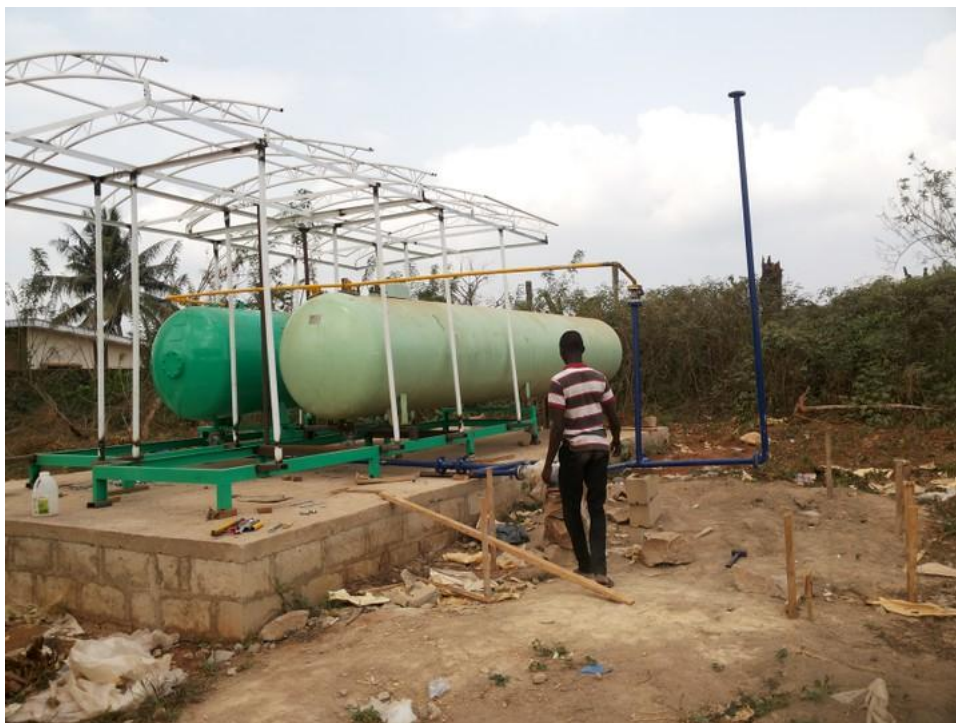
Fig. 1. Sample of a Storage Tank. 40MT. (Please note: It could be elevated or based like this pix base on the size of the land and F.E.E.D)
